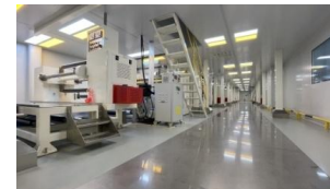
Clean Room, Overall 10,000 Class, Local 1,000 Class
